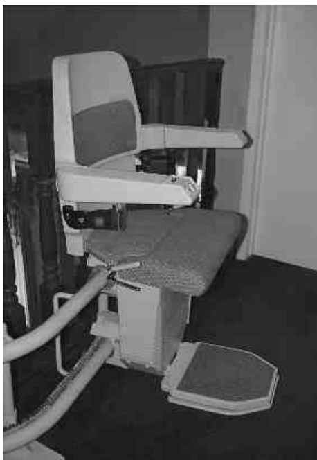
Stair lift at top of stairs on landing
