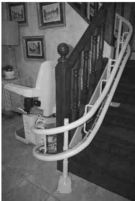
Stair lift at lower station with stairs in view
